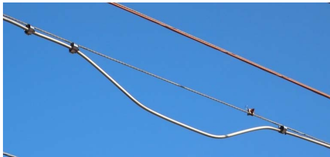
Figure 4 - A cable connection is often characterized by a pronounced dip near a utility pole
