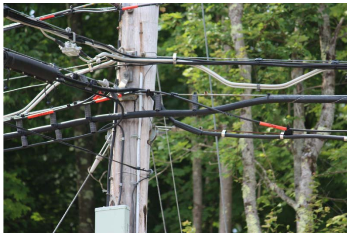
Figure 9 - Fiber-optic cabling along with other technology types
