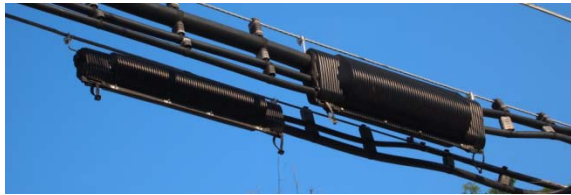
Figure 2 - Telephone utility infrastructure can be identified by black cases or "splice cans"
