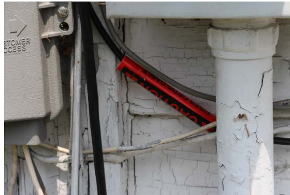
Figure 8 - Sheathing of fiber-optic cable
