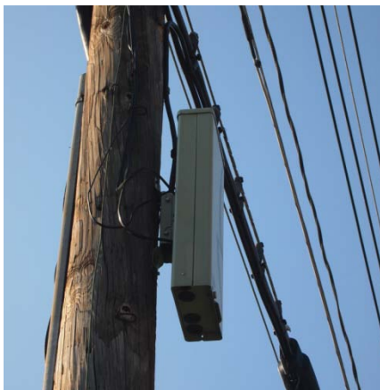
Figure 3 - Flat cables lead from an intermediate cabinet on a utility pole connect a "splice can" and customer NID or network interface device
