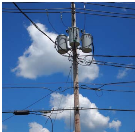
Figure 1 - A utility pole in Keene showing a typical setup: telecommunications service wires are located on the lower section of a utility pole. Power is always located at the top. A distinct safety area allows for maintenance, upgrades, and other work.
